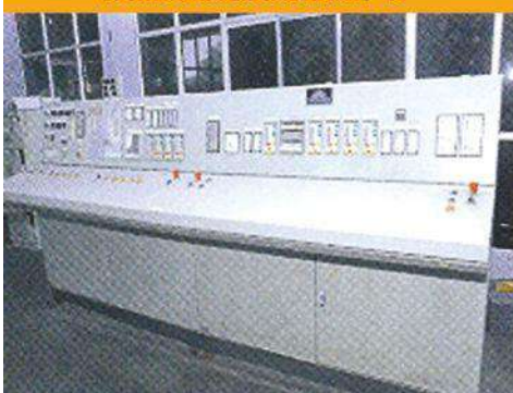
The fully computerised control room of Hardboard Plant - 3
